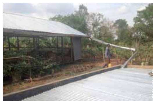
Figure 1: Rooftop rainwater harvesting with gutter and tank
