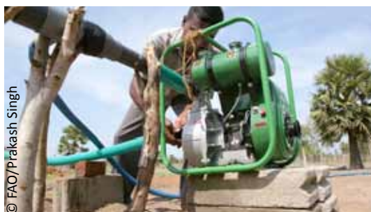
Figure 2: Pump to access water from the tank
